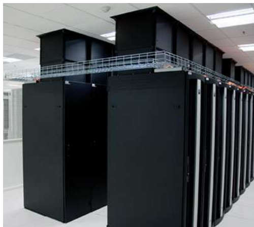
Cooling with Cabinet Containment
